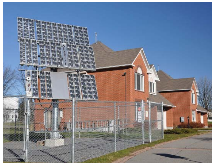
A solar concentrator will be used to provide electricity to the CCHT Reference House in late 2010 as part of the SUNRISE project.
